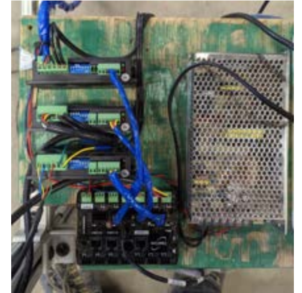
Completed Electrical Component Board
